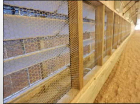
Tunnel shutters in partially closed position
