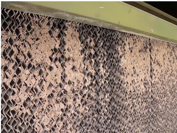
Clogged pads restrict airflow and reduce cooling capacity
